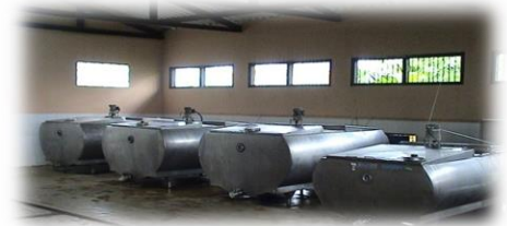
BANTUAN COOLING UNIT
